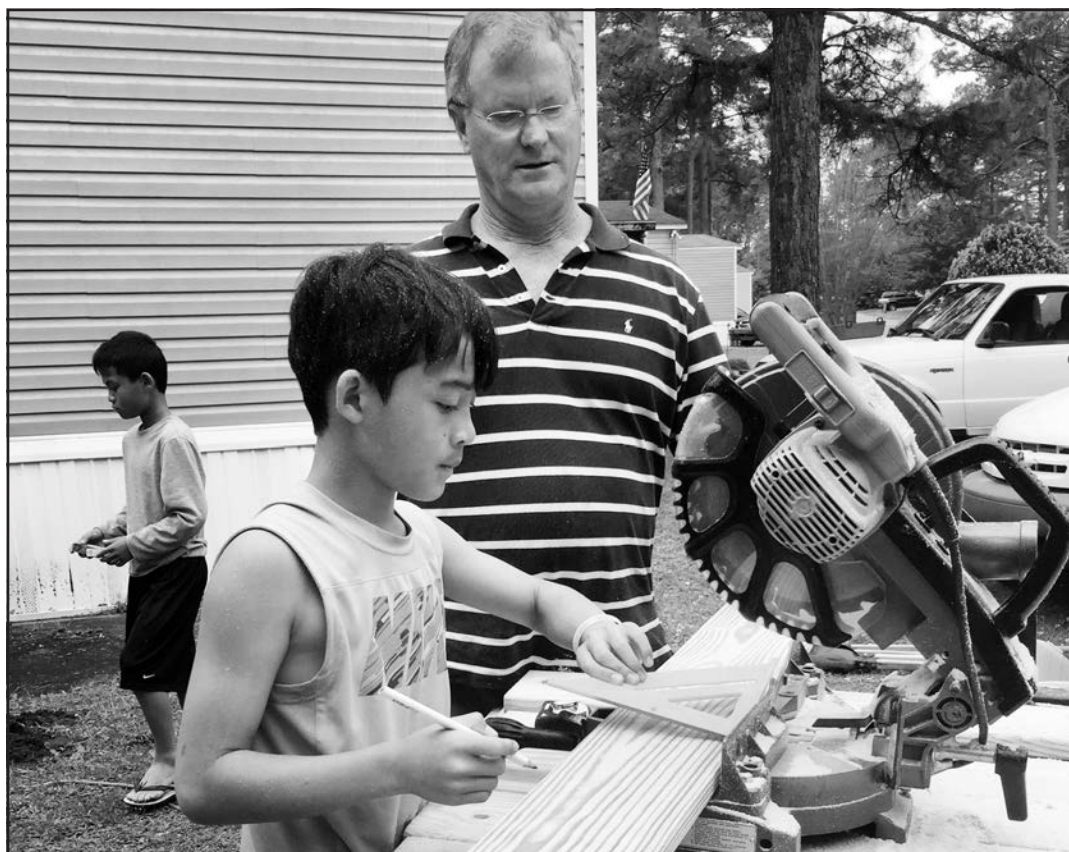
Volunteers from First Baptist Wilmington pass on knowledge to the next generation of ramp builders as they work together on a client's ramp in New Hanover County. Below, David Faircloth, second from left, and members of Mebane First Baptist Church's Handyman Ministry build a wheelchair ramp for an Alamance County client using funds from NCBAM's ARPA/PTRC Grant.
